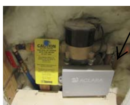
Main water line - Upgraded service pipe to street
