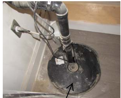
Sump Pump - Storm Water Management System
